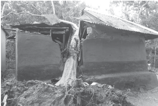
House Damage at Kharagpur I Block in Paschim Medinipur District
