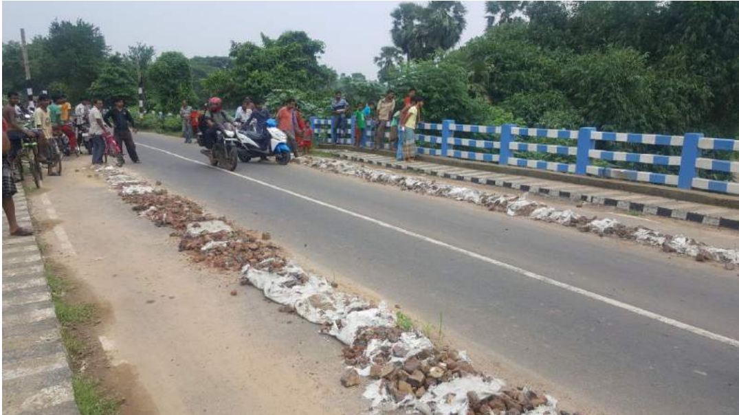
Bridge Damaged at Udaynarayanpur, Howrah
