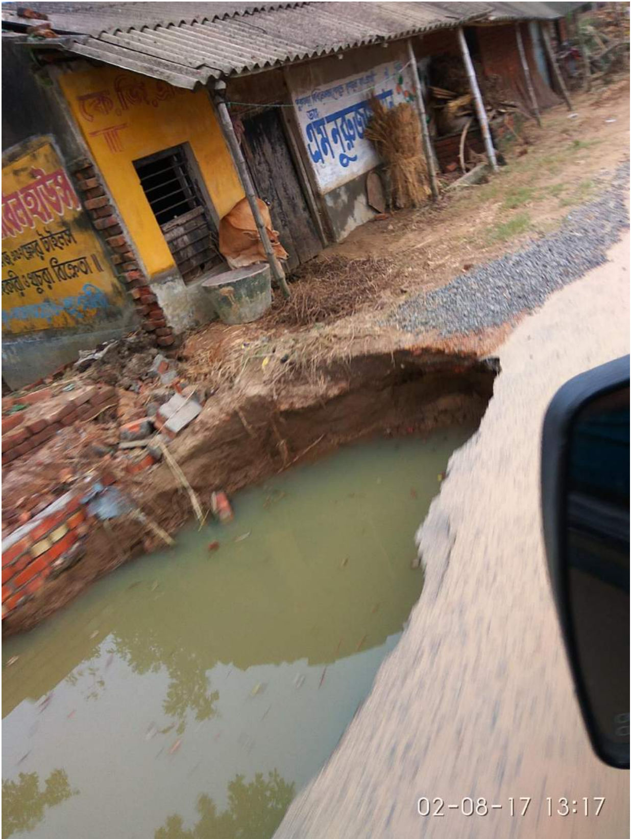
Figure 1: Road Washed away at Arunda GP, Khanakul 1 block, Hoogly districts.
