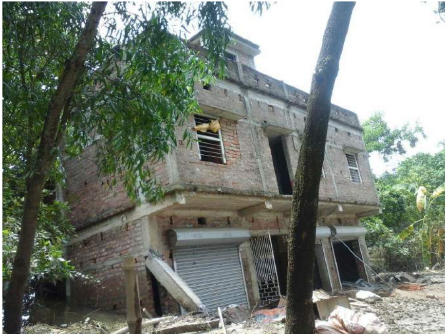
House Damaged in Hooghly
