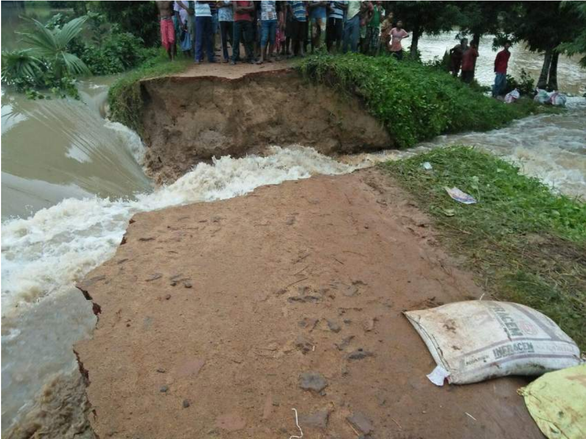
Village Road Damaged at Howrah
