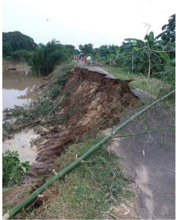
Road Damaged in Hooghly
