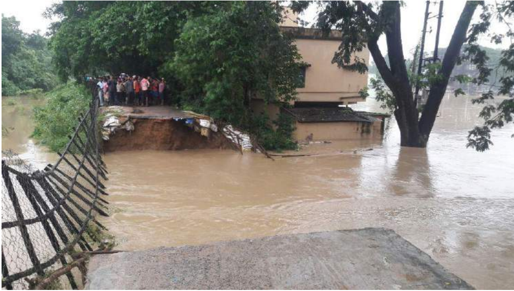
Road Damaged in Hooghly
