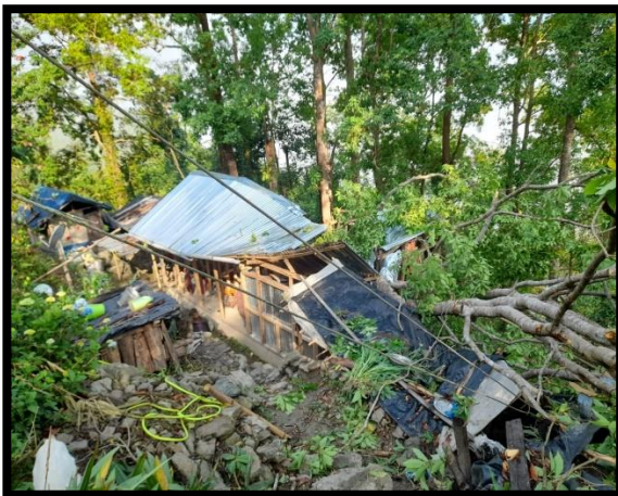
Damage to houses due to heavy wind of at Bhalukhop GP, Kalimpong-I on 21.04.2023
