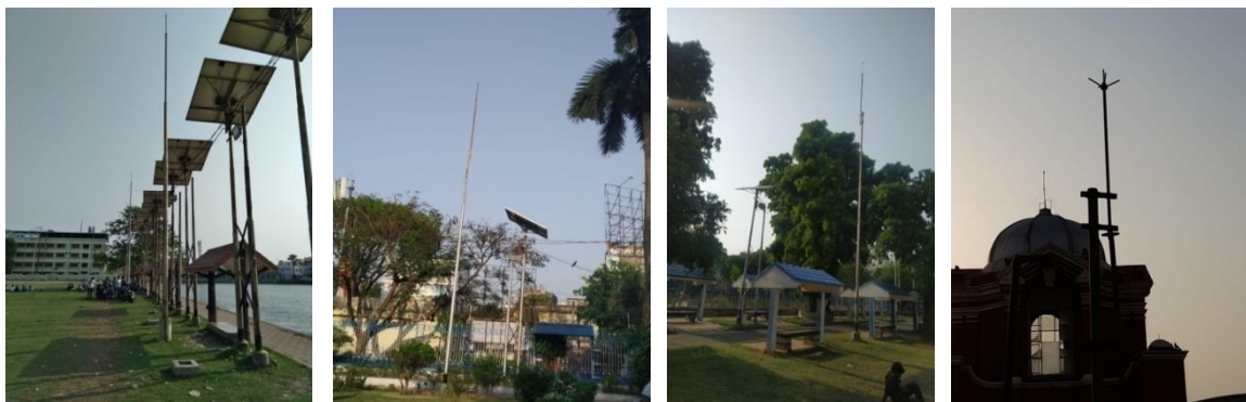
Photo 4.1: lightning arrester in different parks and CMO building of KMC
